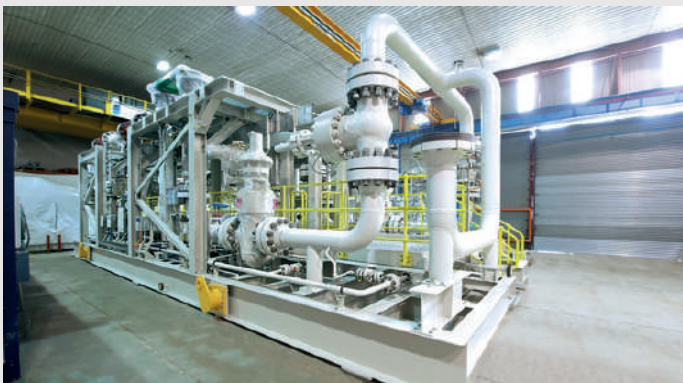
BP Clair Ridge Metering Package (UK Offshore)
